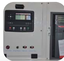
Control Panel & MCB
